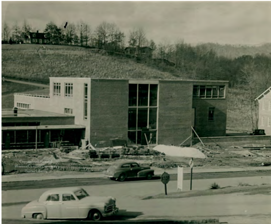
Hunter Library under construction in 1953. Photo used by permission of Hunter Library, WCU
